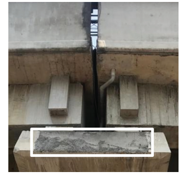
(e) Anchorage recess filled with poor-quality concrete
