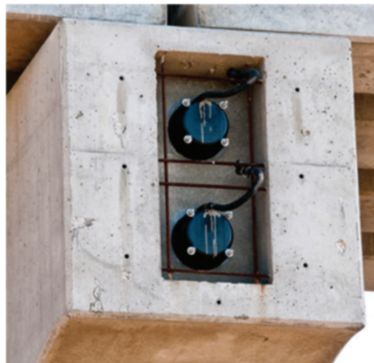
(b) Non-metallic anchorage caps kept well within the recess to be filled with reinforced concrete
